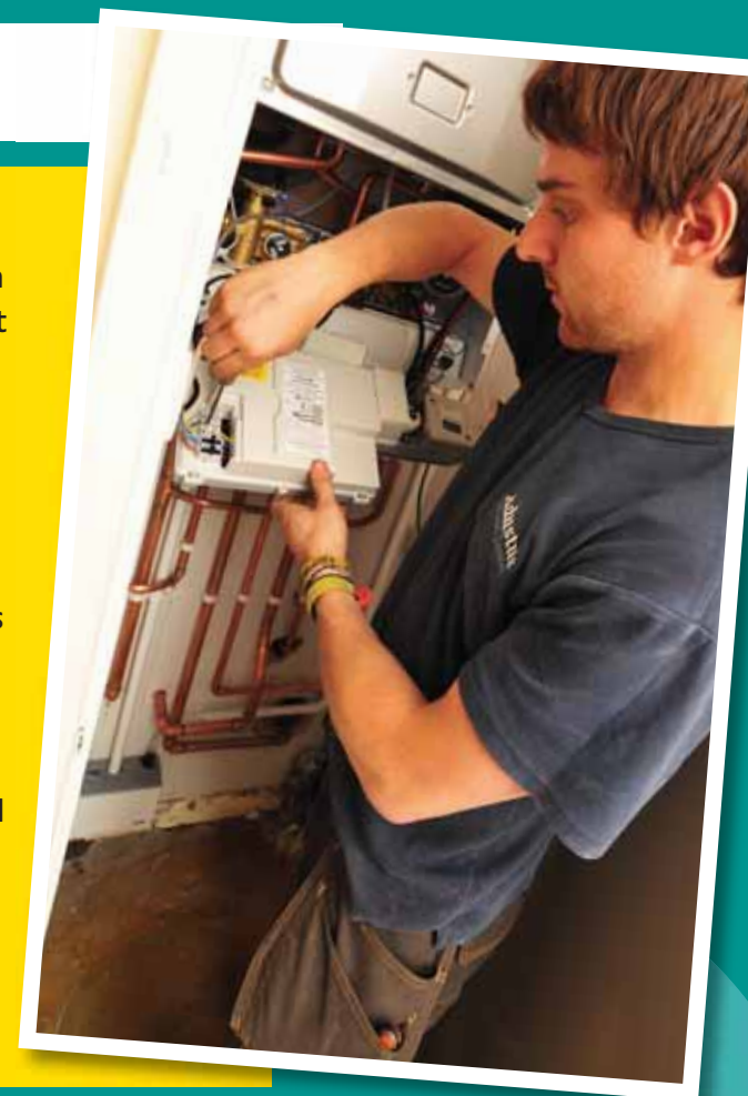
Steve from Adustus Services working on fitting a new boiler in Hellesdon, Norwich
