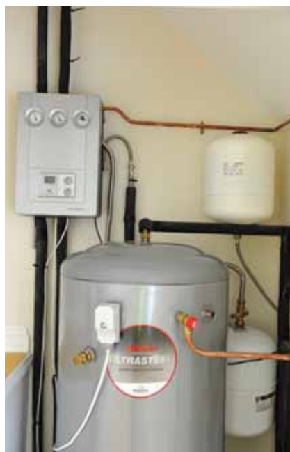
A brand new heating system
